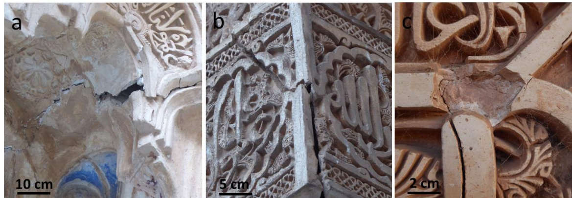
Fig. 2. Decorative gypsum plasterwork (yesería) at the Alhambra fortress (Granada, Spain) showing crack formation and material loss, evidencing the need for compatible replacement materials.
